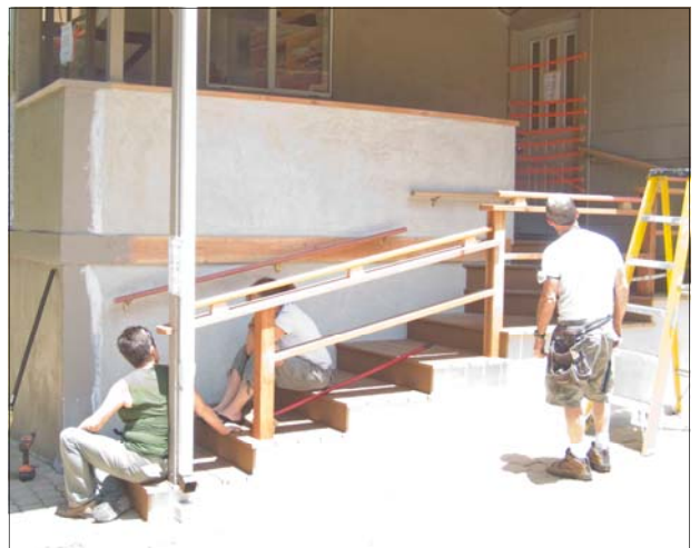
The remodeling of the Sangha House garden entrance and stairs is near completion! The project will make the area safer and easier to use.
